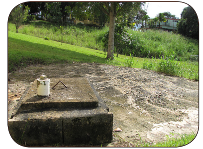
Keep septic tanks sealed.
